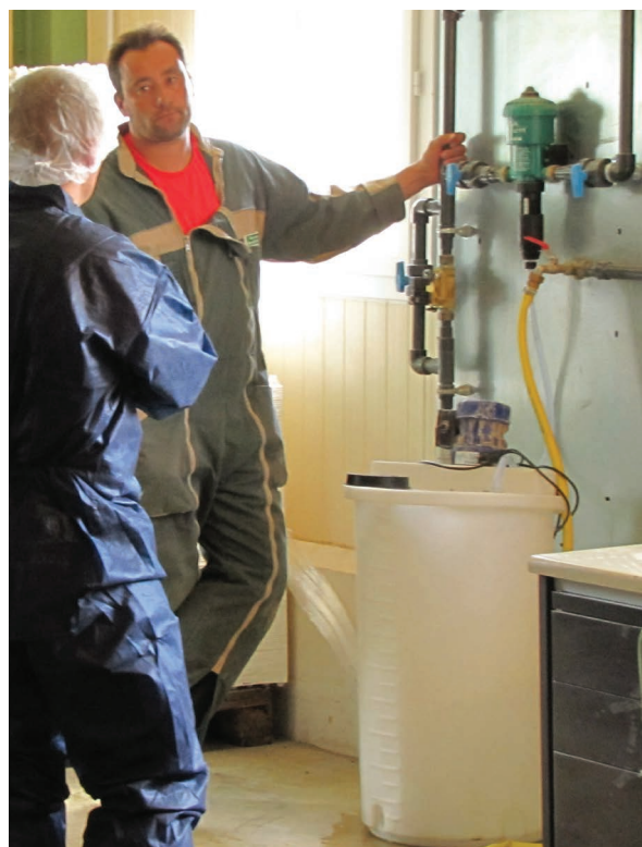
Adhere to Good Practice standards when administering Exzolt through dosage pumps.
